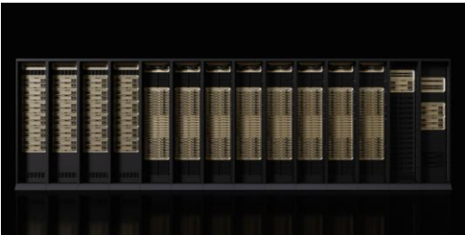
Next-Gen AI Data Center
