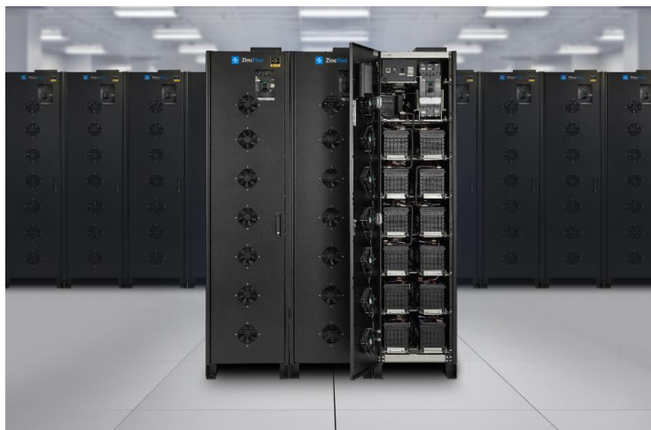
Figure 1: BC 2 UPS Battery Cabinet in data center setting
